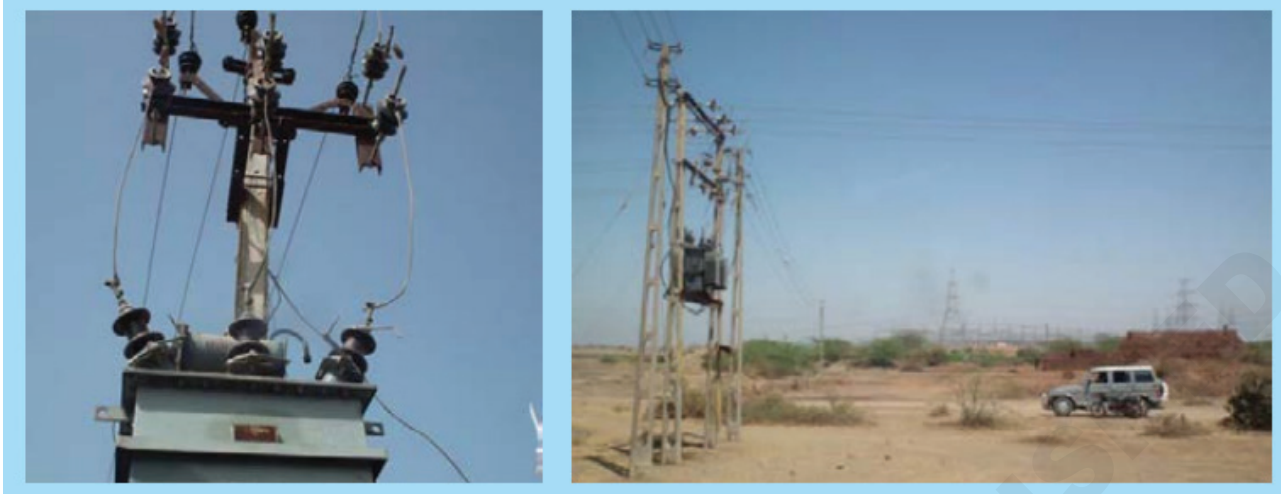
a Distribution transformer on pole
