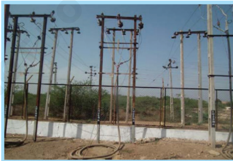
c 11 kV lines emanating from 33/11 kV substation
