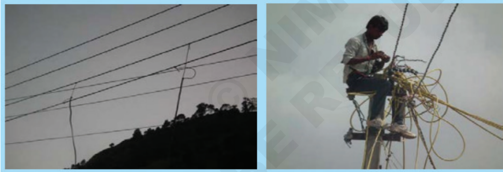
a Tapping of 0.4 kV line
